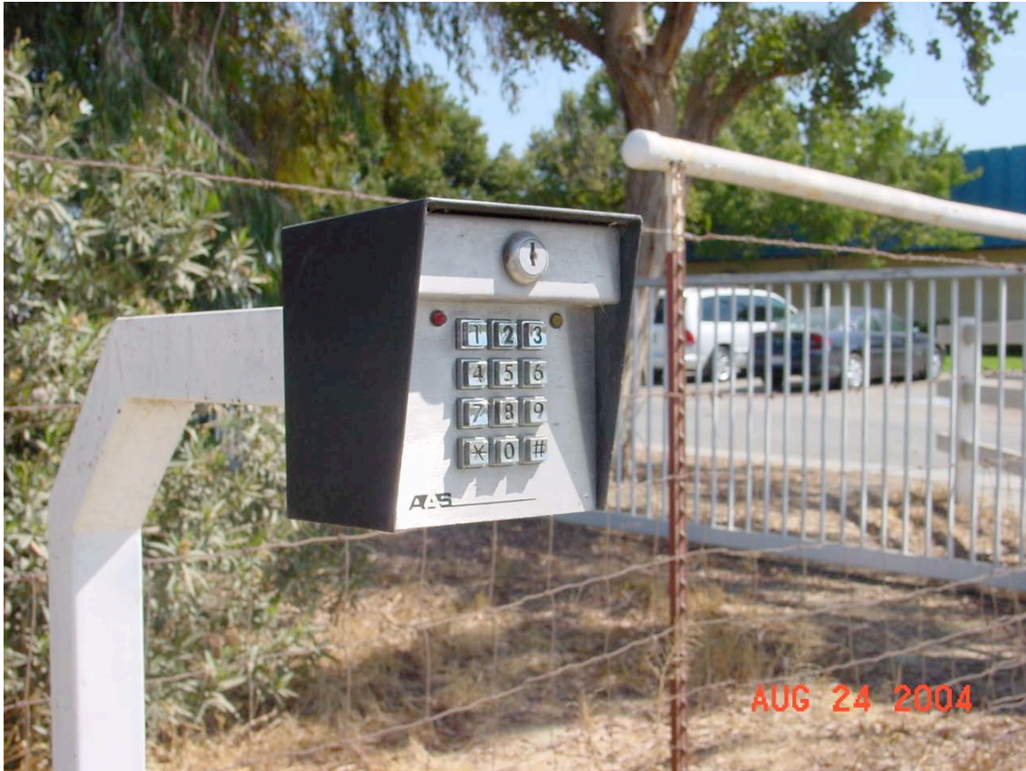
Picture 8. Keypad to control entry through perimeter gate.
