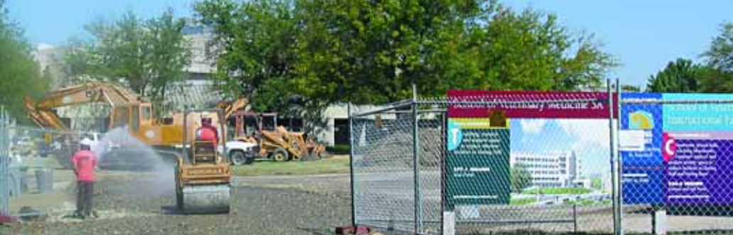
Construction of the $27 million Veterinary Medicine Instructional Facility (VMIF), located between the Veterinary Medical Teaching Hospital and Schalm Hall, began last July.
