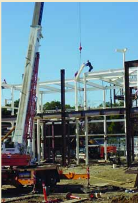
January 2005: The skeleton of the VMIF grows as steel beams are guided into place.
